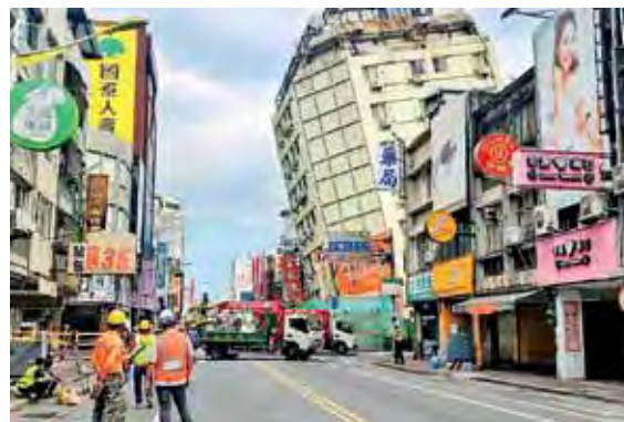
Hualien, Taiwan The Full Hotel building, which had been previously damaged in the April 3 earthquake, tilts further to one side after a series of earthquakes overnight.
